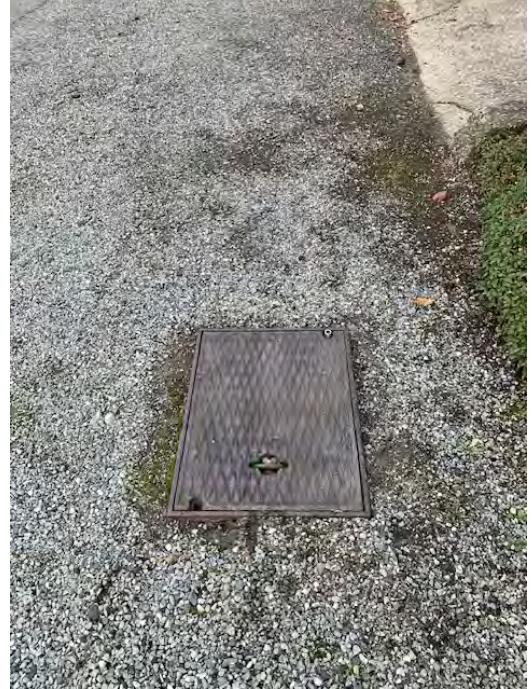
Looking Downstream from Catch Basin – At Point B
